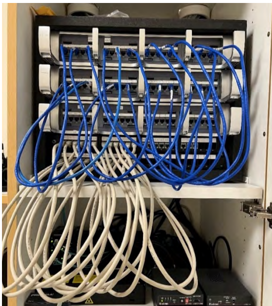
Control Room Patch Panel
