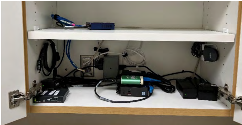
Control Room STC Station Cabinet
